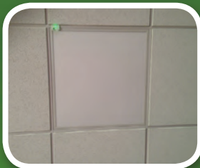
After (fire integrity is maintained)
