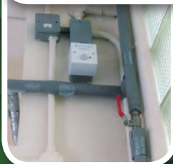
Installation of urinal flush control units should save 129,600 litres of water per year
