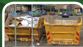
Recolight is a lighting disposal/recycling specialist is managing the project waste in accordance with WEEE legislation
