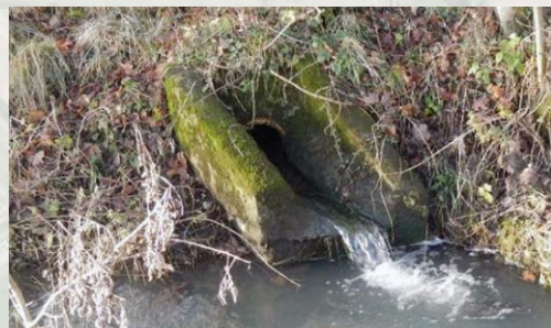
Albermarle Barracks sewage outfall into the Med Burn.
